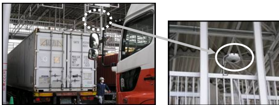
Figure 2-4 An example of a 433MHz-band interrogator installed on a gate.
