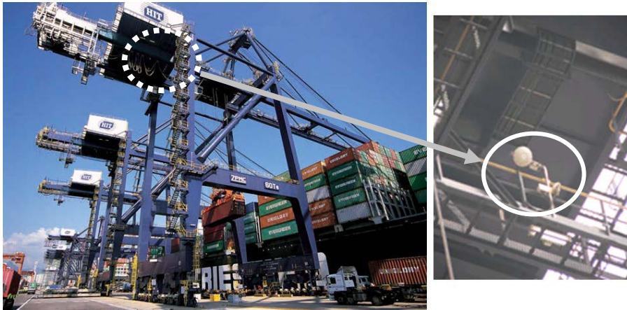
Figure 2-5 An example of a 433MHz-band interrogator installed on a crane at a harbor
